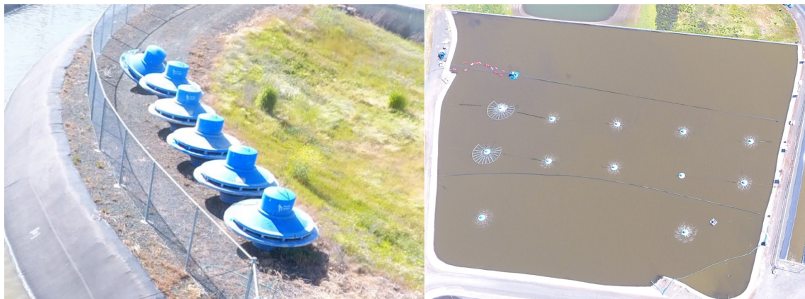
Figure 2) (a) (left) Image of the Blue Frog aerators that are used at the Southeast Treatment Plant. (b) (right) Image of the Blue Frog aerators being used in the south pond at the facility (Eric Luna, 2024).
