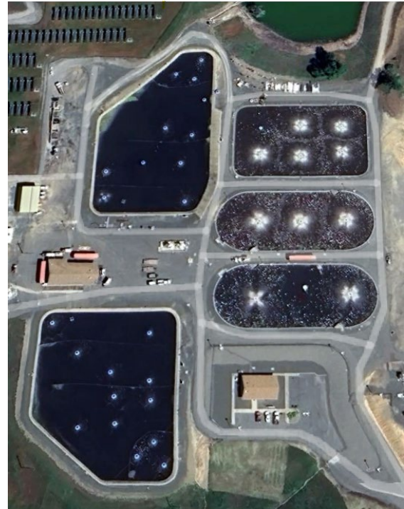
Figure 4) An aerial photograph of Lake County's Northwest Wastewater Treatment Plant. On the right side are the three aerobic ponds. On the left side are the two facultative ponds (Fisher, 2024).
